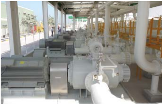
Numerous Twinro pumps installed at a fuel oil terminal in the UAE
